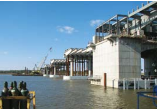
Spliced girders with lightweight concrete were used on the Route 33 Bridge over Pamunkey River.
