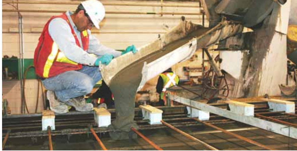
This UHPC has been mixed in and is being discharged from a ready-mixed concrete truck. Photo: Ben Graybeal, FHWA.
