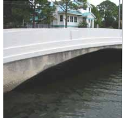
The Shore Drive Bridge was constructed in 1923 by the Luten Bridge Company.
