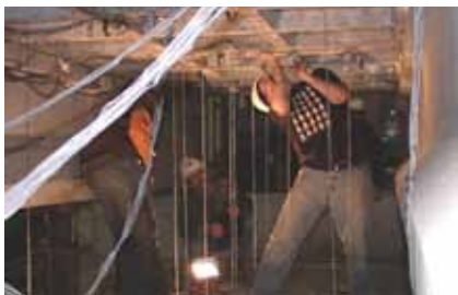
Precast UHPC waffle slab deck panels passed the testing program shown here at Iowa State University and are part of the design for a Wapello County bridge to be constructed in 2010.
